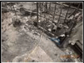
Extension cord taped to the floor
