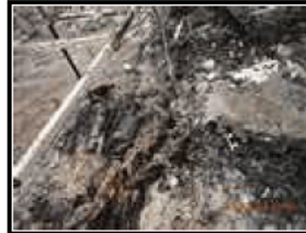
Extension cord running to power strip
