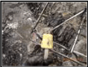
Cord that was plugged into floor box
