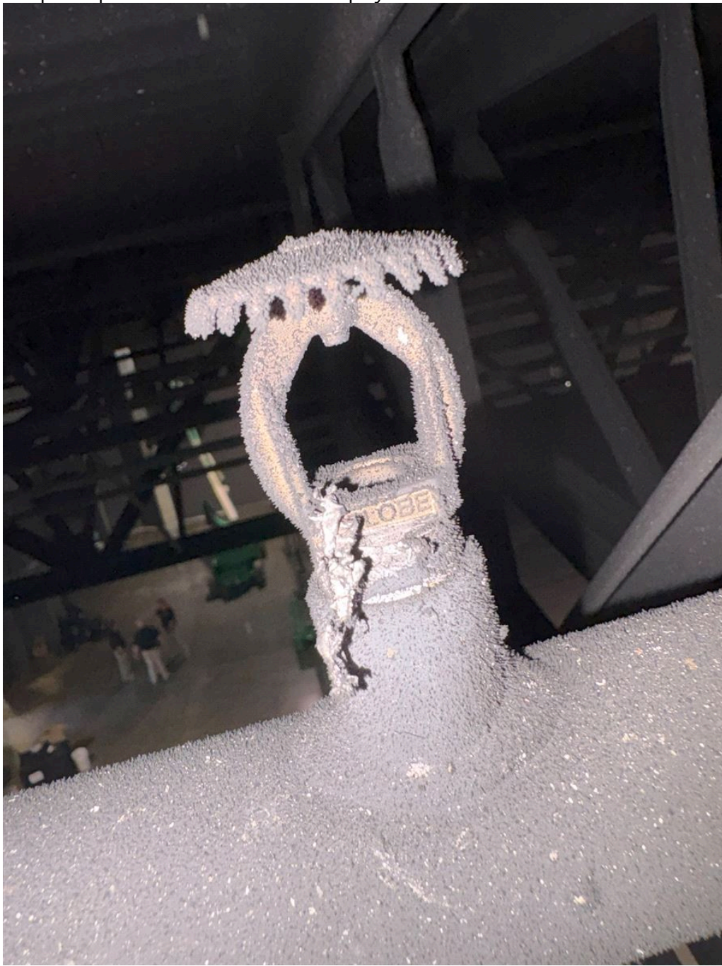
Title: photo of close up of a sprinkler head that has been deployed above where the fire occurred
