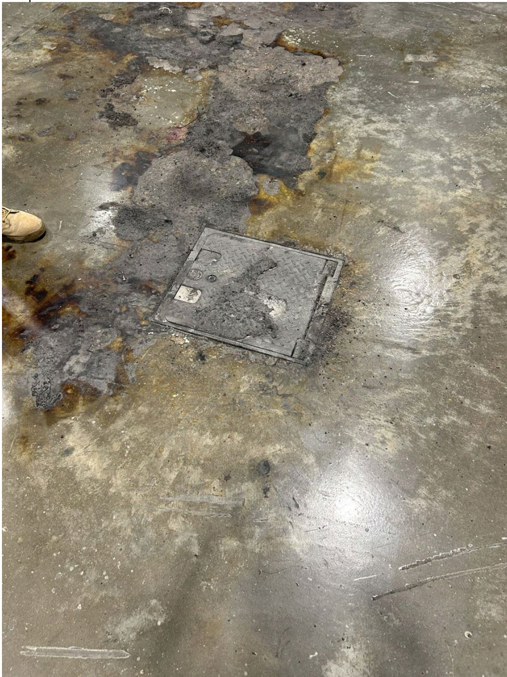
Title: photo of close up of where fire occurred in trademart
