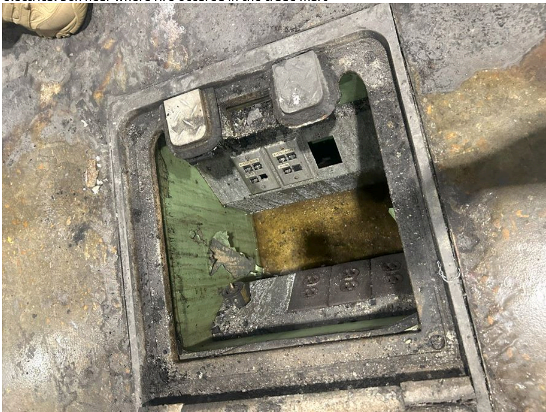
Title: photo of electrical box near where fire occurred in the trade mart
