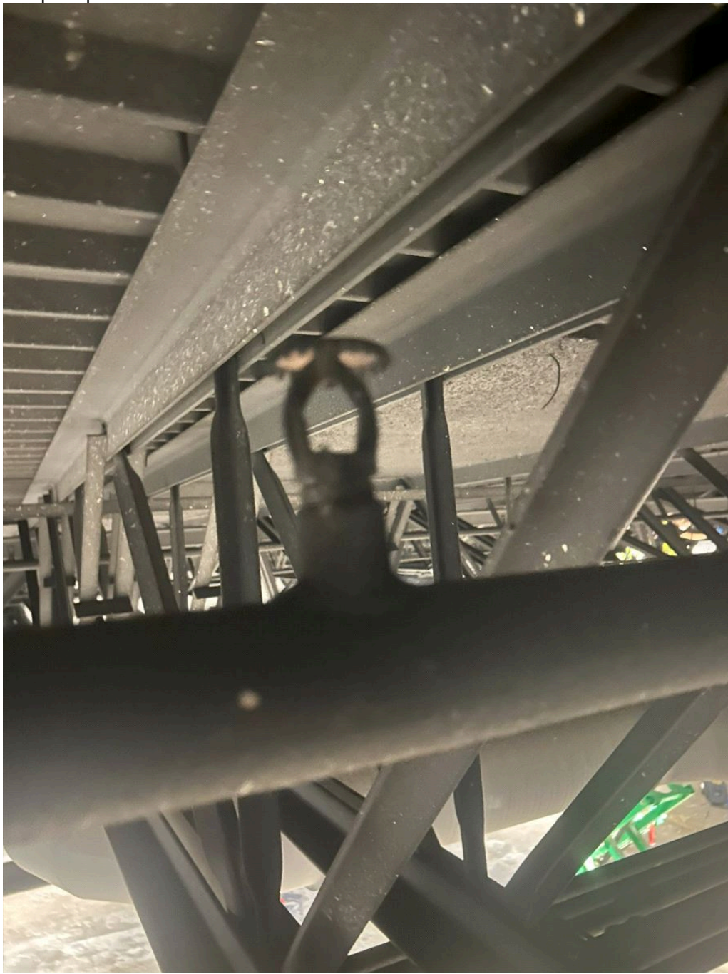
Title: photo of close up of sprinkler head above where trade mart fire occurred
