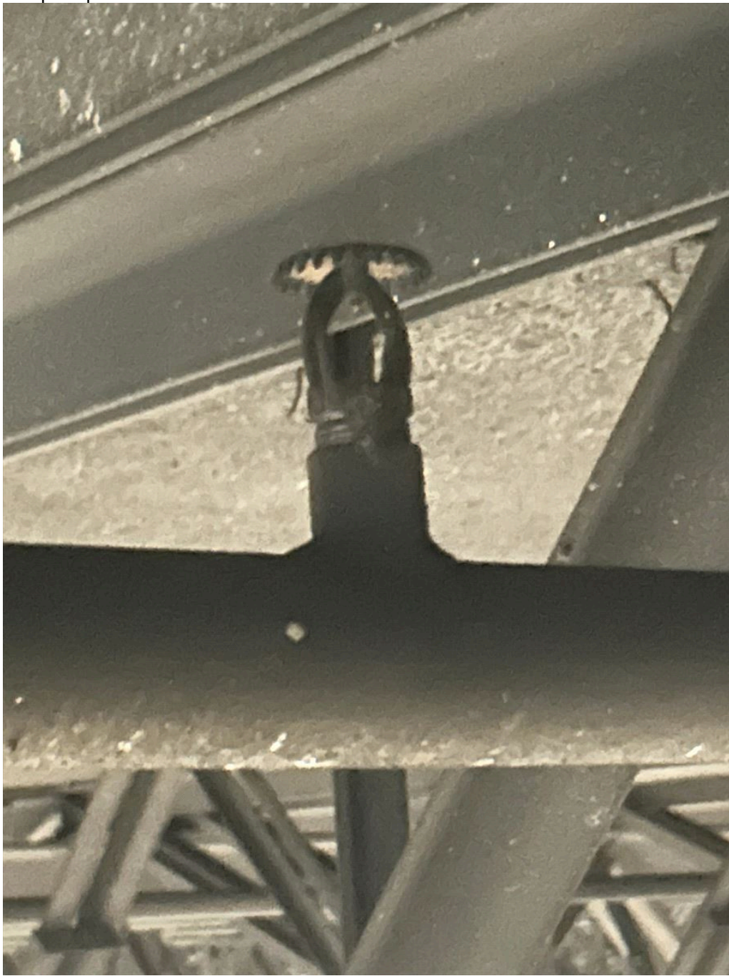
Title: photo of close up of sprinkler head above where fire occurred
